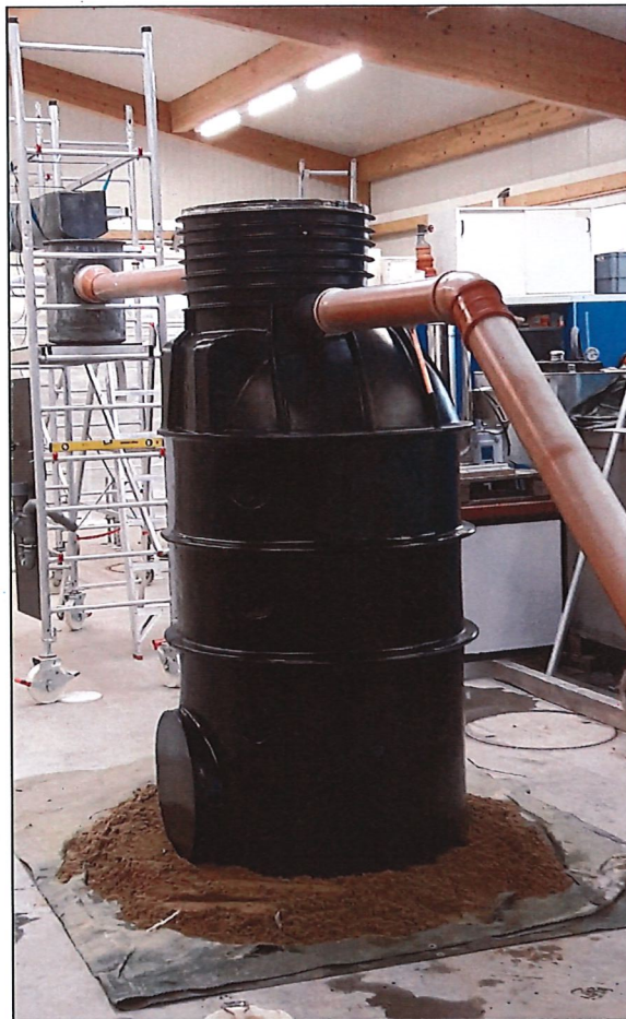
Figure 1: Separator before testing
